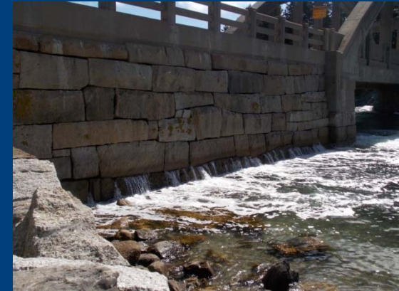
Tidal water penetrating through Northwest wing wall near High tide
