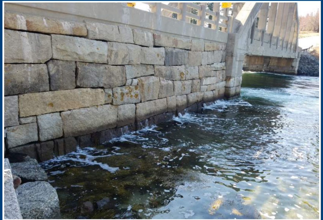
Existing masonry voids and water penetration
