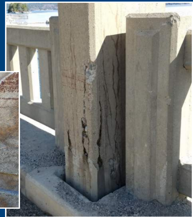
Deteriorating Concrete Hanger
