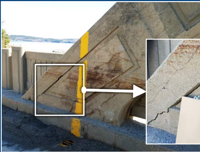
Cracked Arch Rib End (Knuckle)
