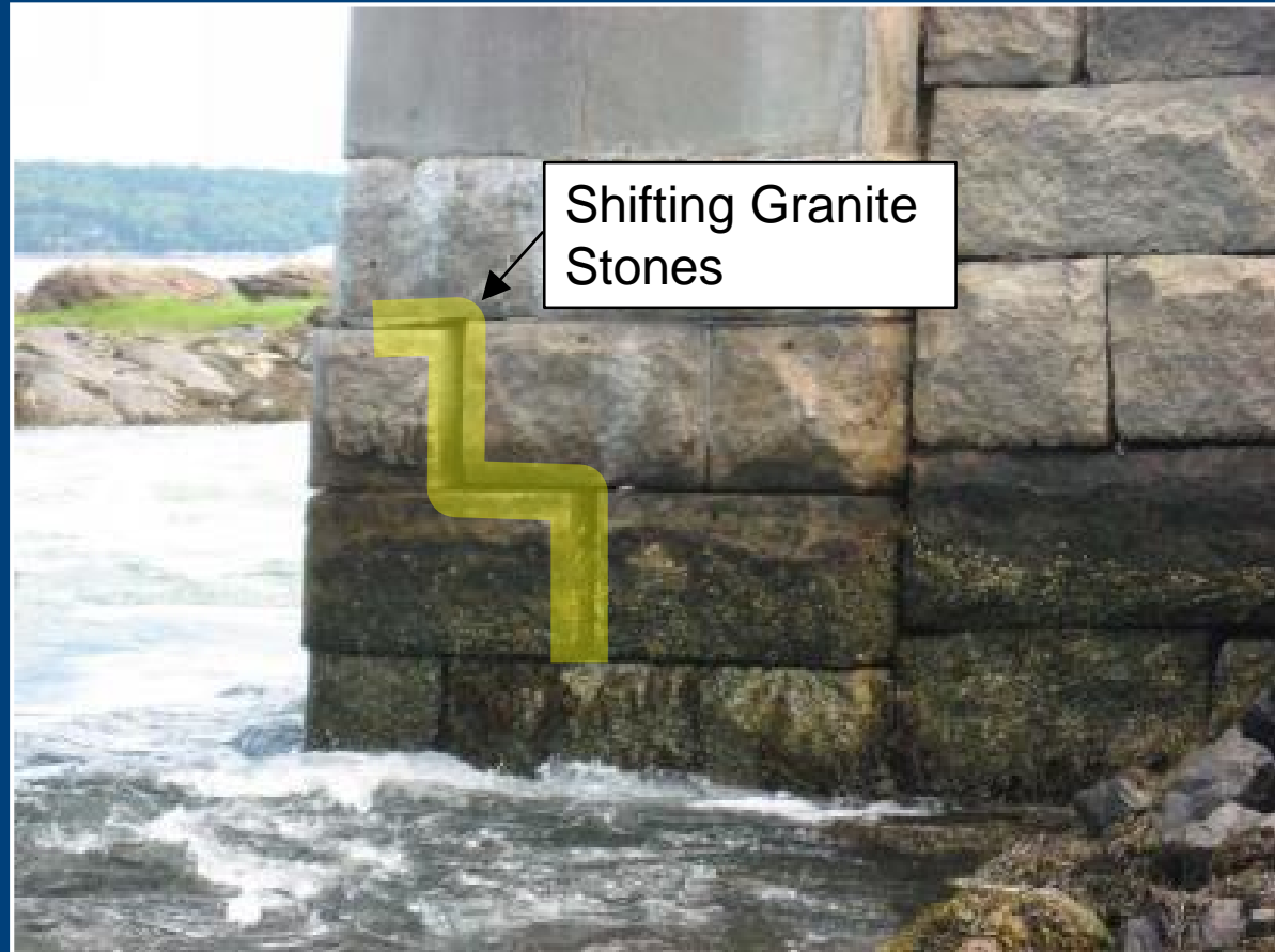
Settling & Shifting Masonry
